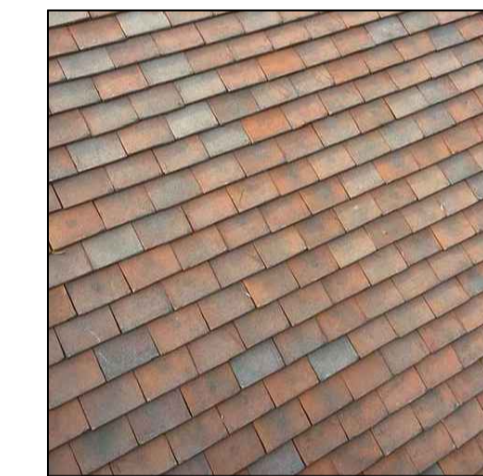
Clay Plain roof tiles to match existing style of tile seen on Farm House.
