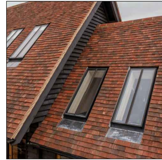
Anthracite Grey conservation style roof lights proposed to provide natural light to first floor landing area.
