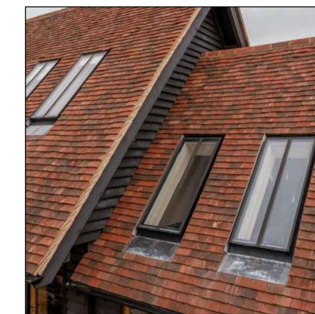
Anthracite Grey conservation style roof lights proposed to provide natural light to first floor landing area.
