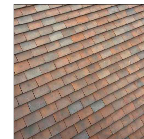
Clay Plain roof tiles to match existing style of tile seen on Farm House.
